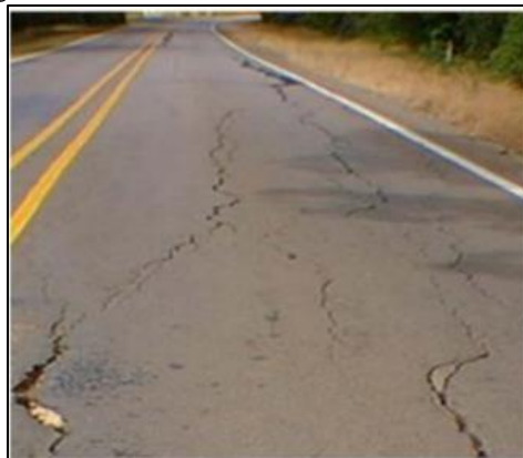
Figure 6 Longitudinal cracking due to subgrade shrinkage adapted from Sebesta [19].
