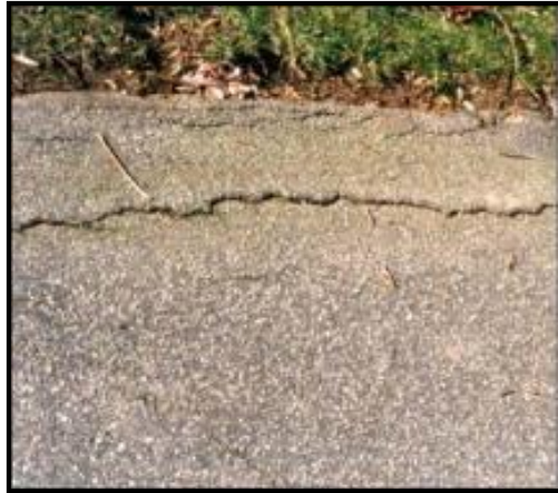
Figure 8: Edge Cracks due to Shrinking of Soil, adapted from Sebesta [19].
