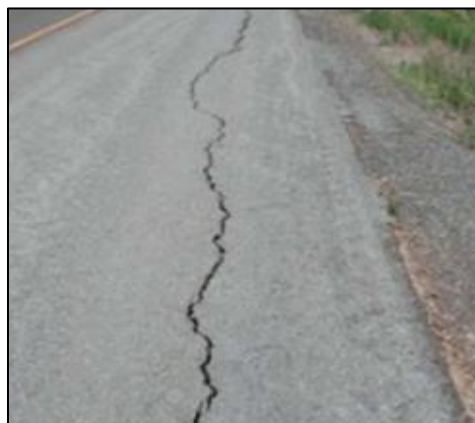
Figure 7: Longitudinal cracking due to pavement fatigue adapted from Scullion et al. [20].
