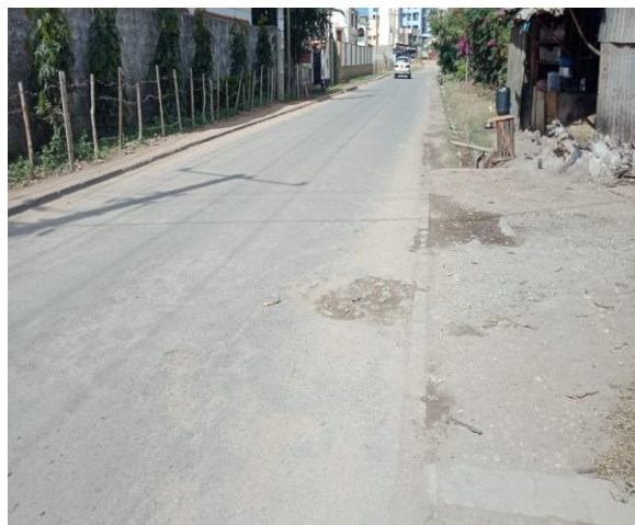
Figure 3.1 Distresses along the surveyed road
