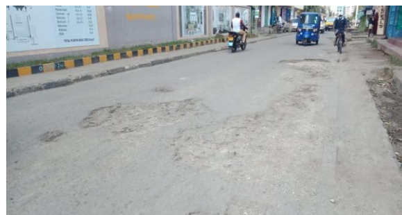
Figure 3.1 Distresses along the surveyed road
