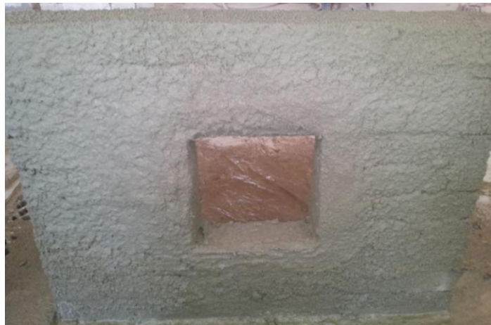
Fig- 9 Covered the strip of steel wire mesh by grout of cement mortar on both sides of wall
