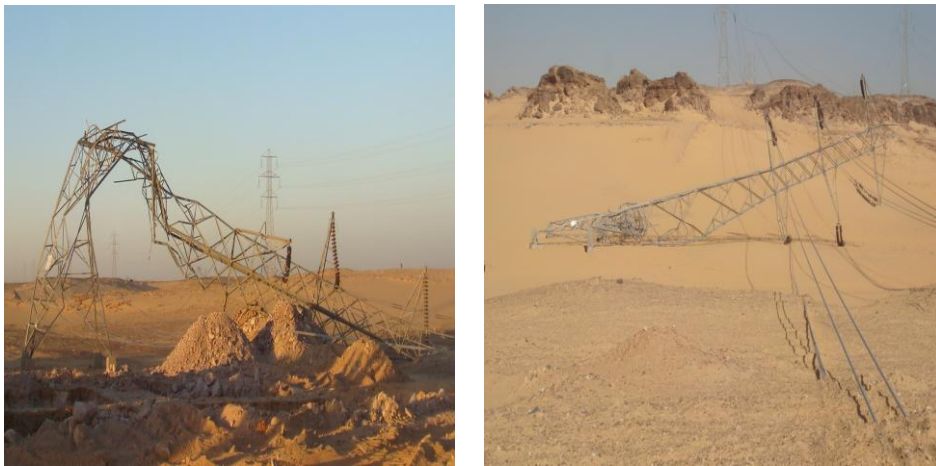
Figure (10) 220 KV real collapsed tower
