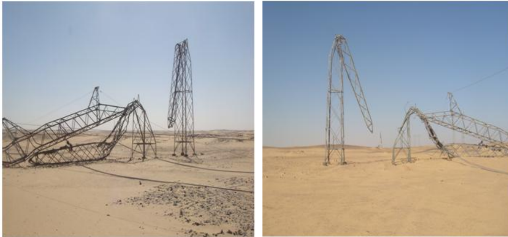
Figure (12) 500 KV real collapsed tower
