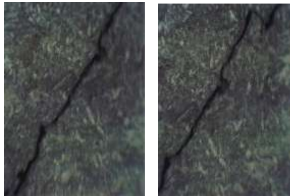
Fig. 9 Cracks within material
