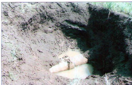
Fig 1. Leakage at RCC pipe and MS Special
