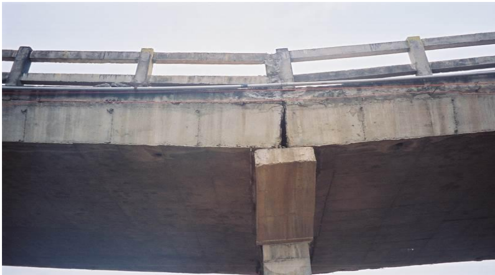
Photo.2. Close view of the settled pier at deck level
