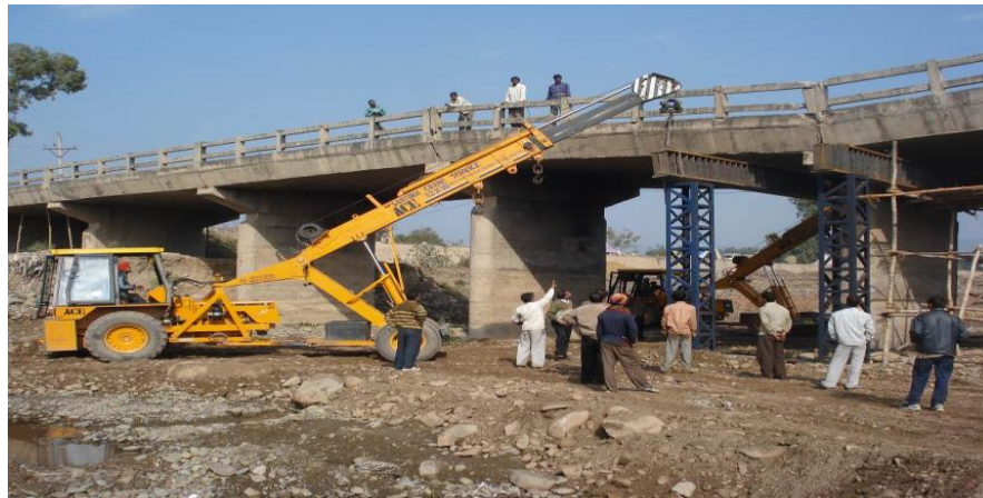
Photo.19. Erection of steel portals on either side of pier of Balad bridge
