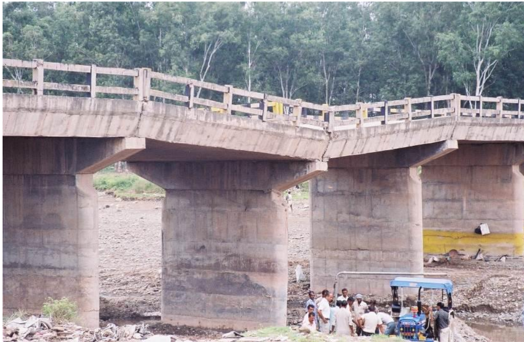
Photo.1. Settlement and tilting of the foundation and pier of Balad bridge
