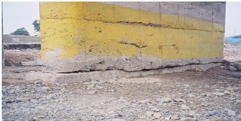
Photo.5. Wide crack at the base of one of the piers
