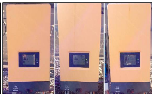
Figure 4: Connected inverters on FSBM
