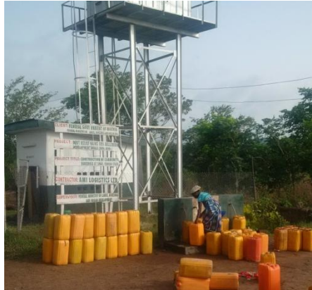
Plate 2 : A borehole with elevated tank located within Shao Township
