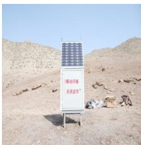
a) Sink node cabin
