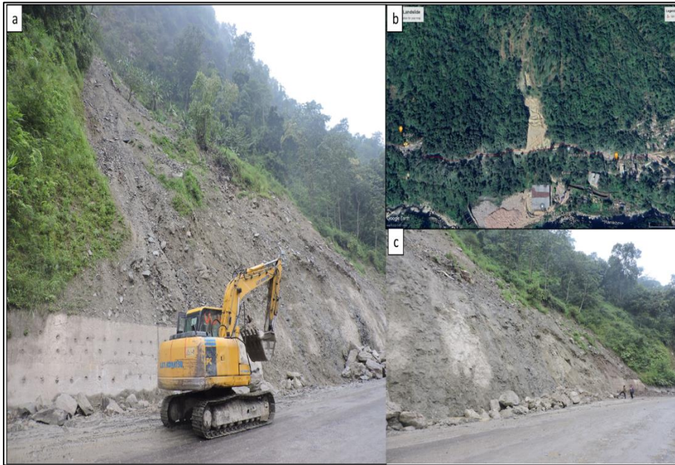
Photograph 1: (a) & (c) showing the side view of the Martam landslide along NH-10, (b) showing panoramic view of Martam landslide (Source: Google-earth image).
